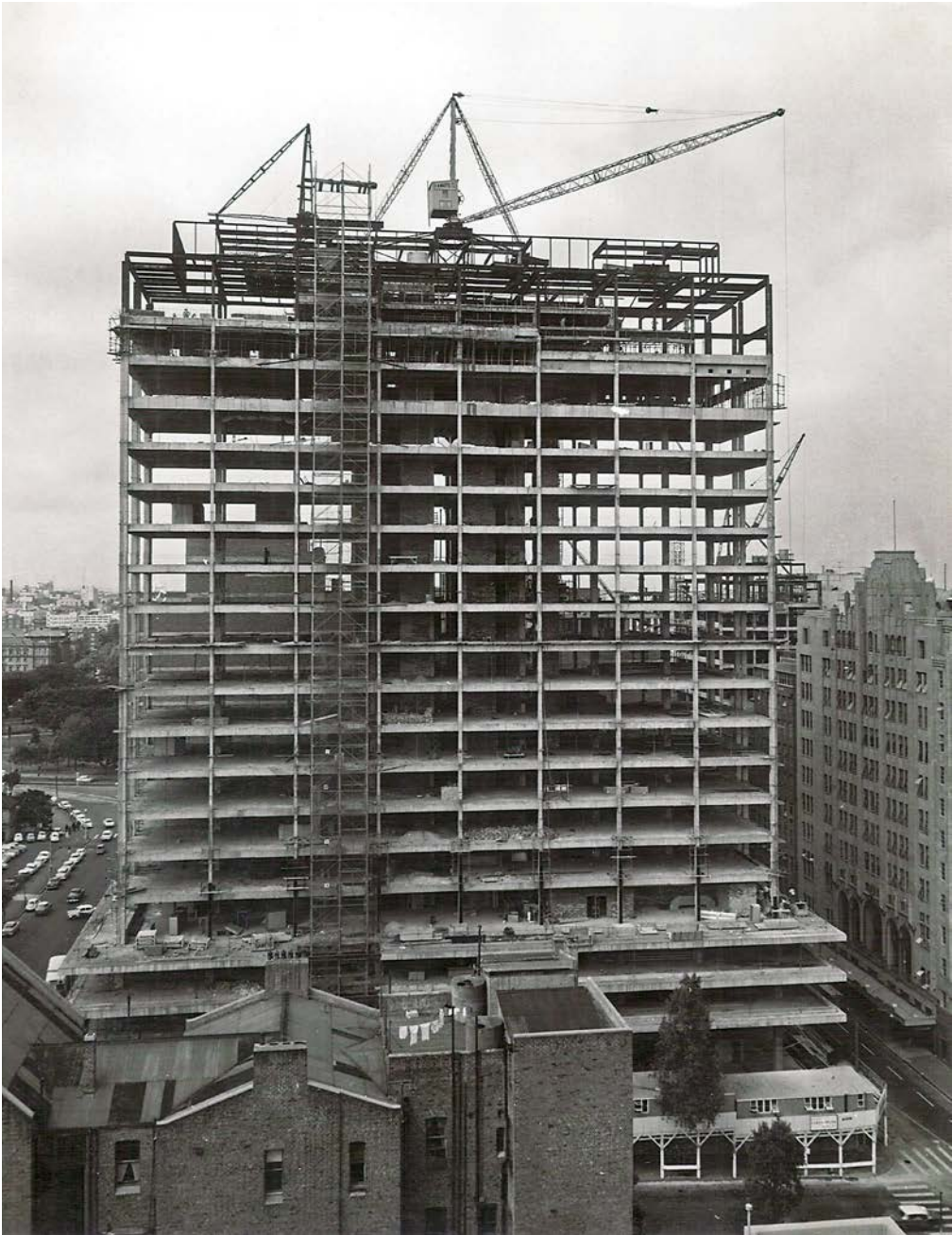
View of building under construction in January 1963. Reserve Bank of Australia Archives. PN-003407.
